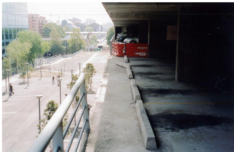
Section of failed barrier
