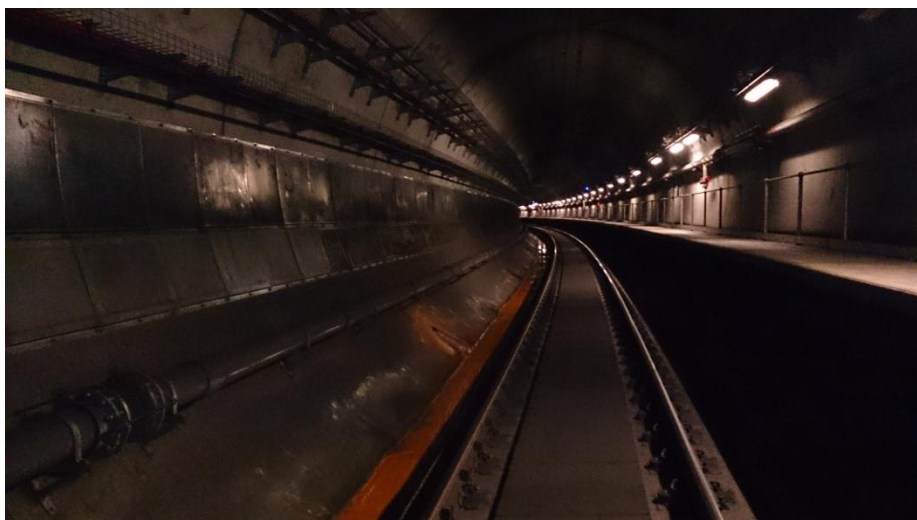
Section of the tunnel, showing the metal acoustic panels on the left hand side. Photo: P Riordan
